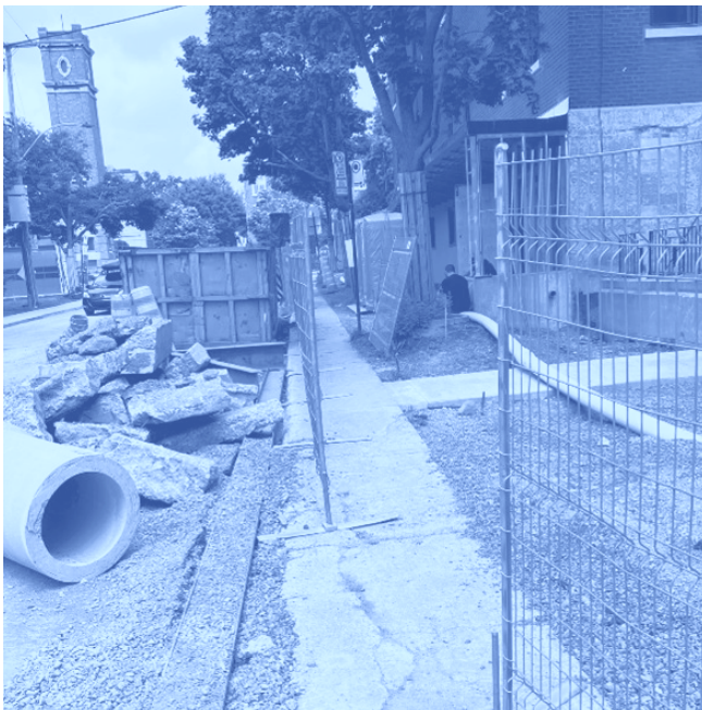
Investigators challenged those in charge of the work on site after noticing glaring deficiencies that put the safety of people circulating near the worksites at risk. Photo credits: Office of the Inspector General
