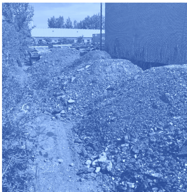
Off-site management of residual granular materials such as levelling or concrete residuals from the demolition of pavements and sidewalks is not adequately controlled on Montréal worksites. In this photo, pavement levelling residuals were disposed of on private property. Photo credits: Office of the Inspector General
